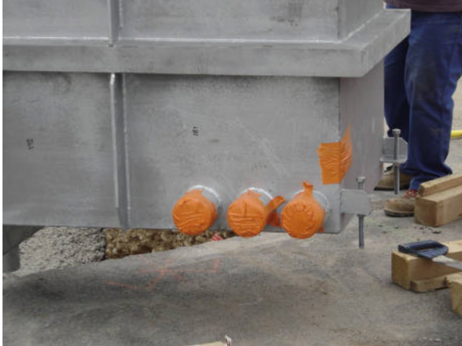
Unused conduits are sealed. Note leveling bolts.
