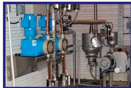
Potable water service unit
